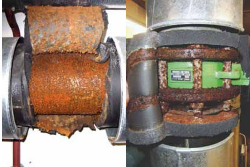
corroding steel pipes
