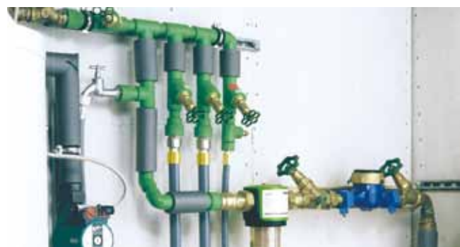
House connection station
