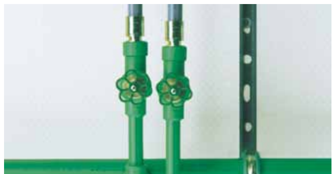
aquatherm grey pipe connection
