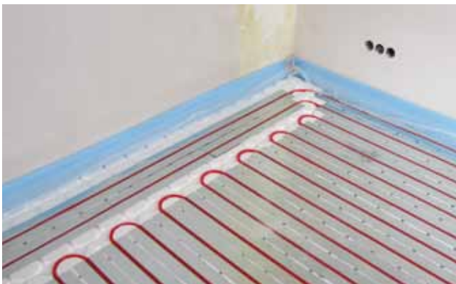
Completed heating system 25
