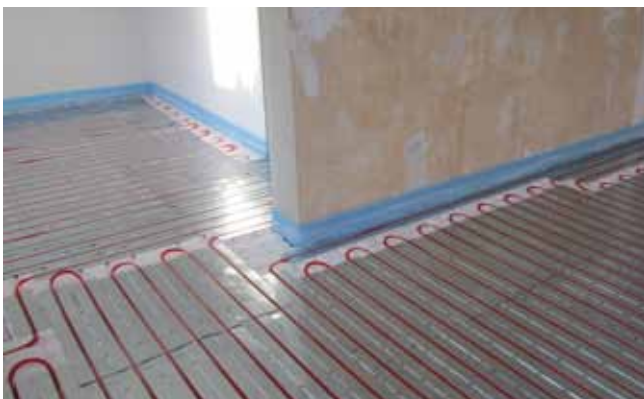
Completed heating system 25
